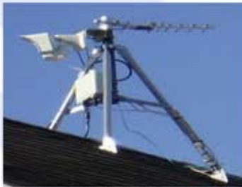
MeshCam™ rooftop installation Featuring Mobotix M12 camera
